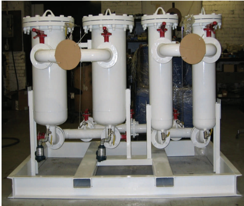
Skid mounted filter package
