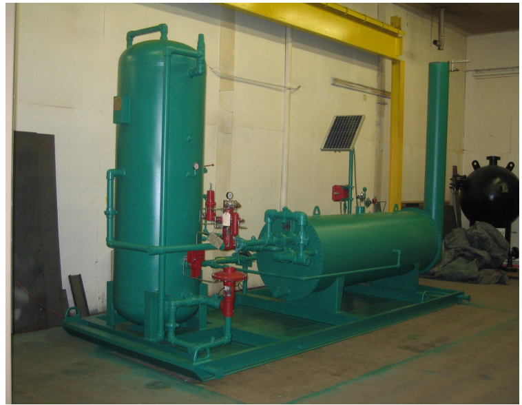
GPU unit 1440 psi vertical separator
