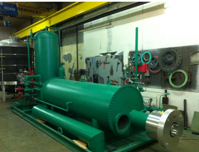
1440 psig skid with 750,000 BTU Heater
