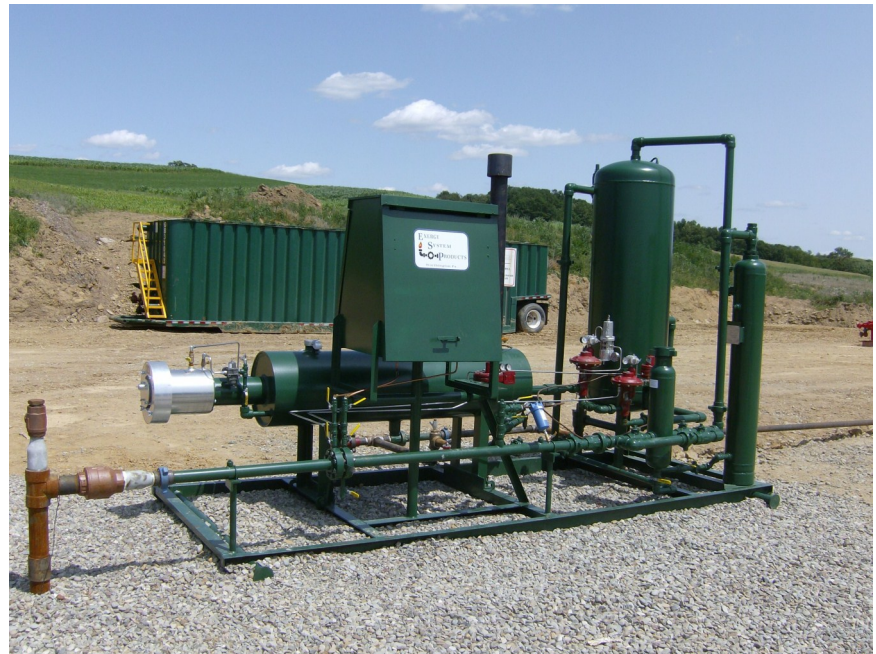
2500 psig skid with heater, separator, filter and meter run
